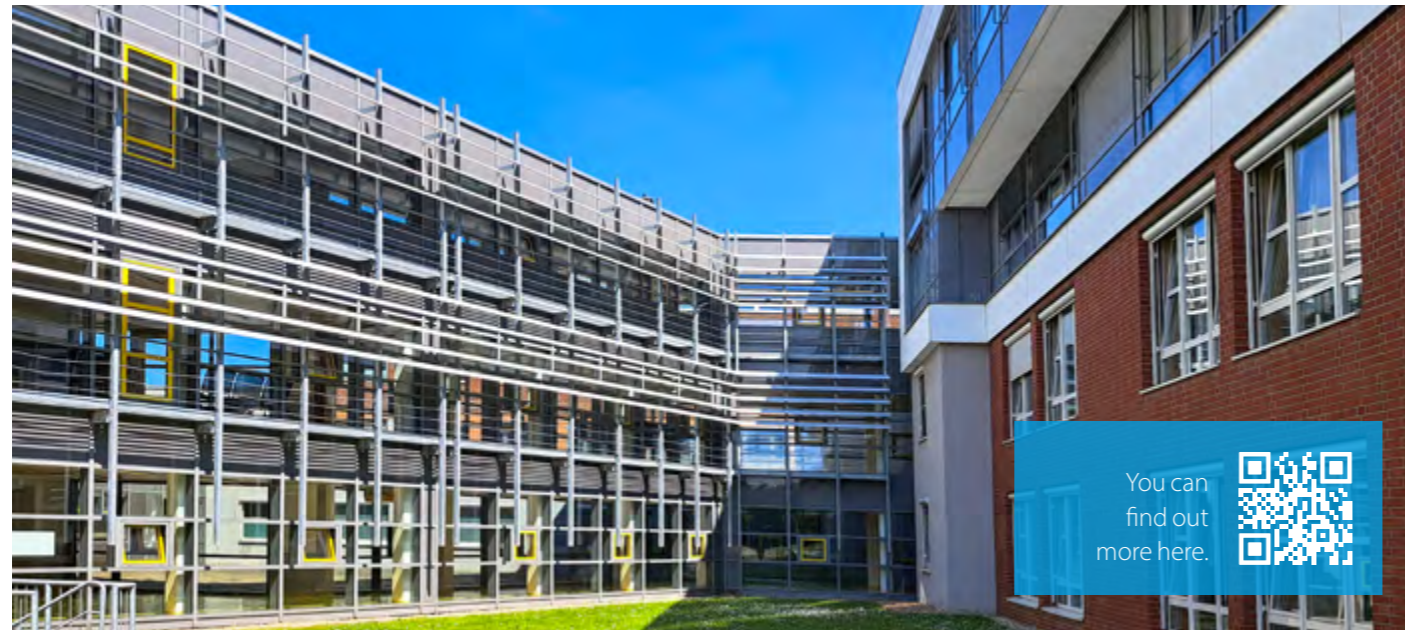
The Hermann-Josef Hospital in Erkelenz received a four-cabinet IS-1 Edge Row Type 4 system with two SideCoolers mounted in a row and, as the centrepiece of the system, the technology rack with Powerbox from SCHÄFER IT-Systems
