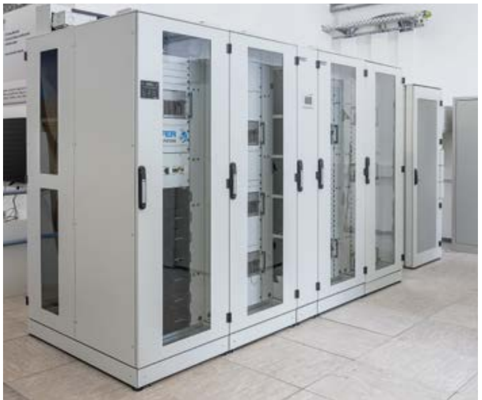
Tested cooling system: closed loop concept with typical data centre components
