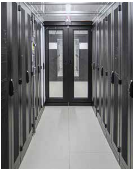
View inside a cold aisle enclosure
